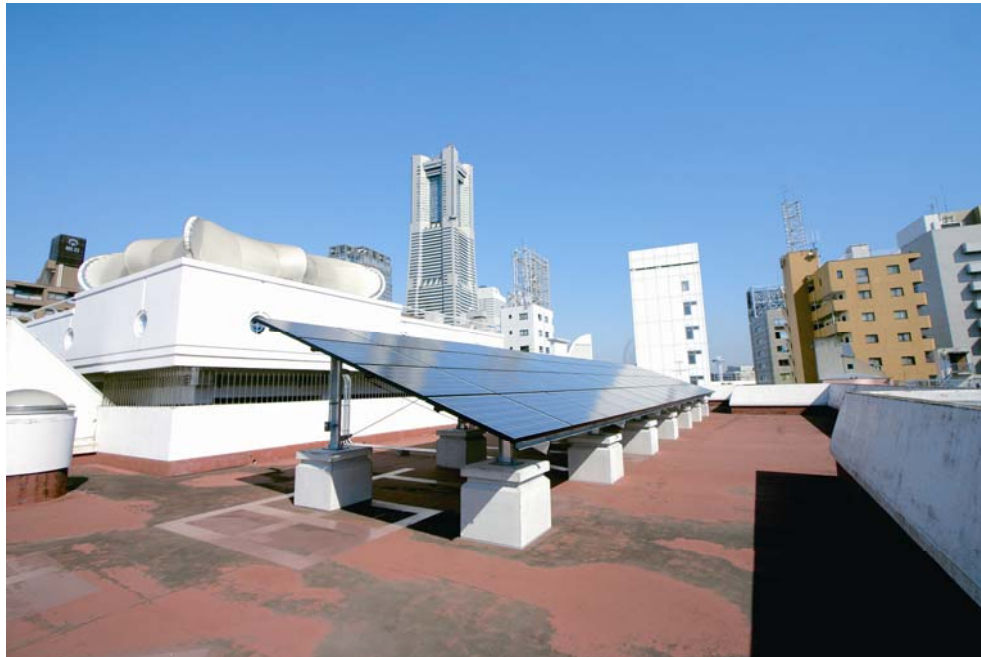
The Solar Panel at Honcho Elementary School
