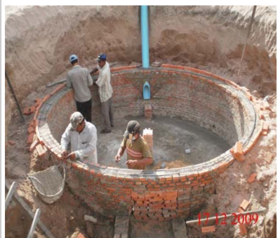
Construction of Biogas in Phnom Penh with the help of HELP-O from Sri Lanka, an associate member of CITYNET
